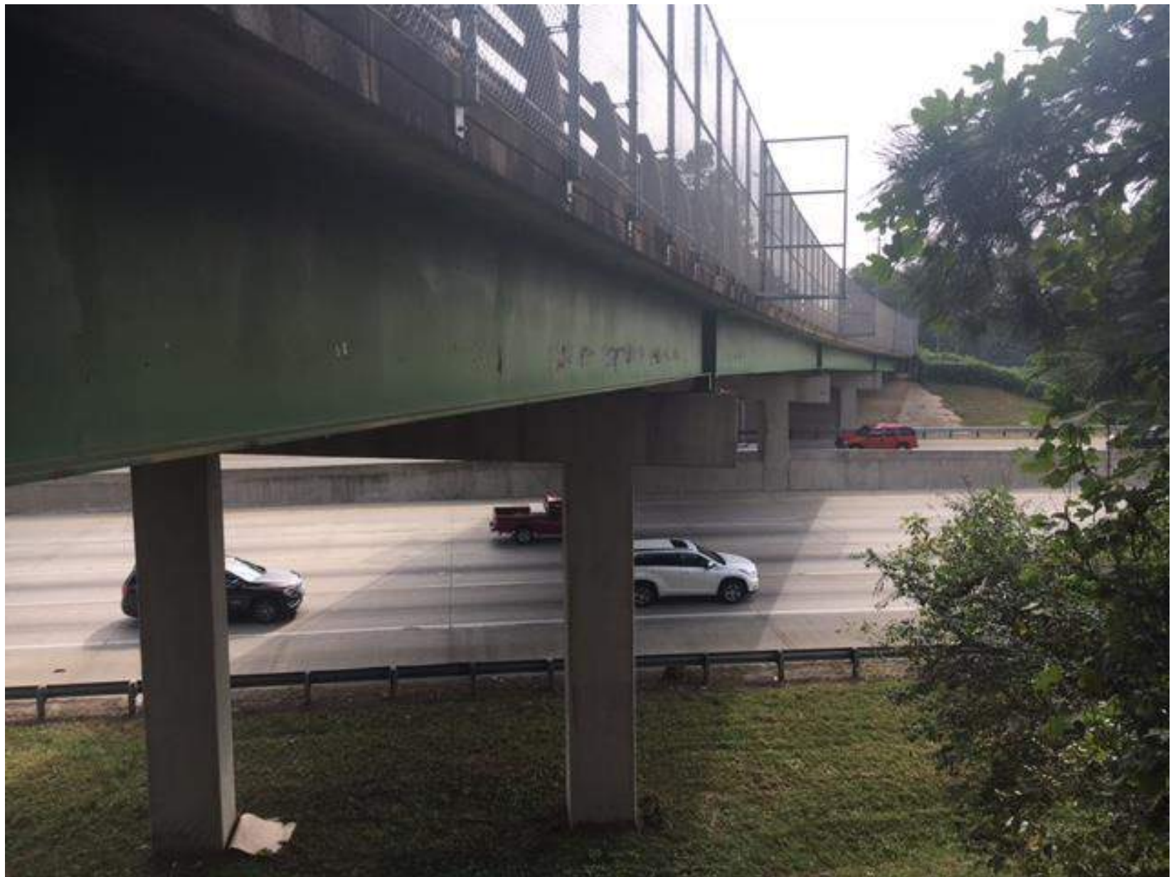
FIGURE 1 Kimball Bridge Road over SR 400 EXISTING BRIDGE SOURCE: GDOT Bridge Inspection Report
