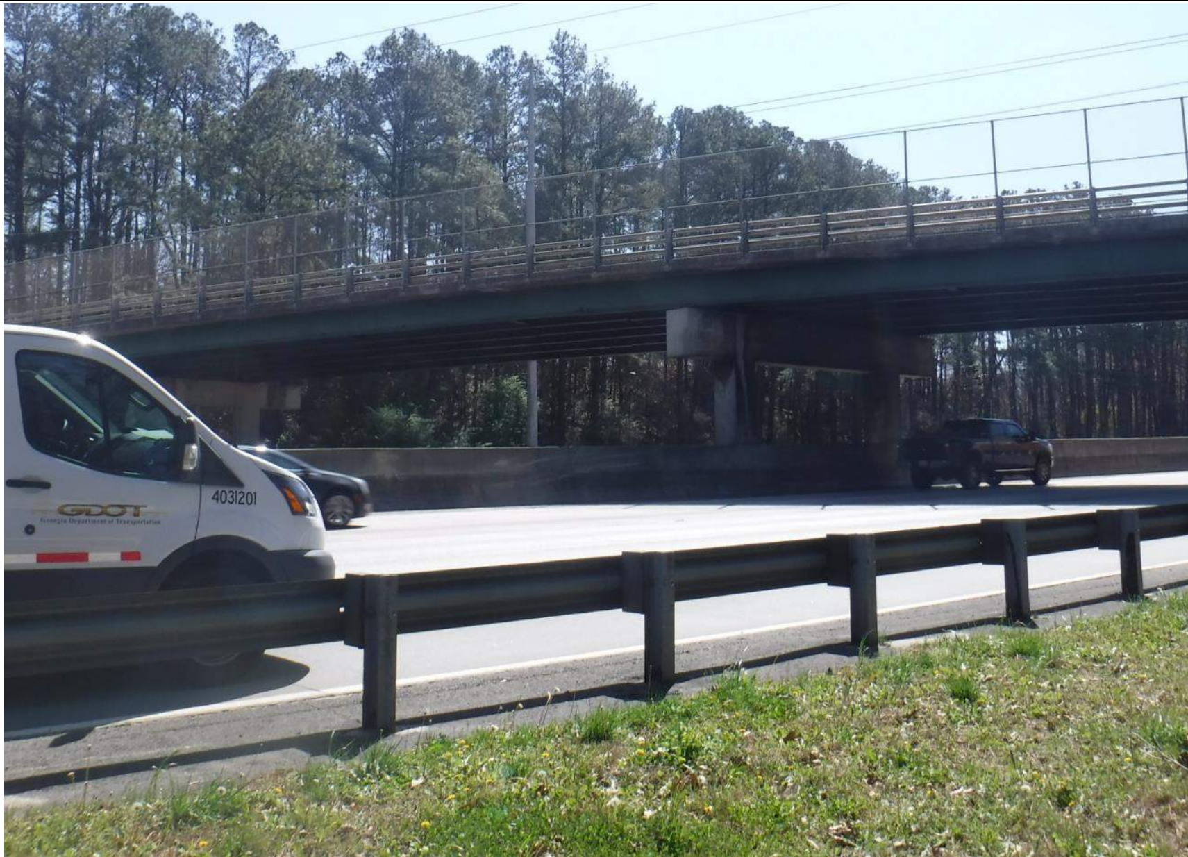
FIGURE 1 BRIDGE 2 – Roberts Drive over SR 400 EXISTING BRIDGE SOURCE: GDOT Bridge Inspection Report
